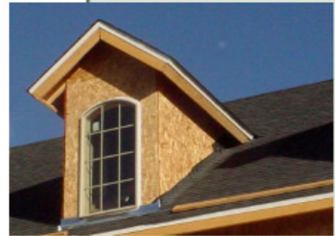
The intersection between the roof and the wall of this dormer should have a good water management strategy.
